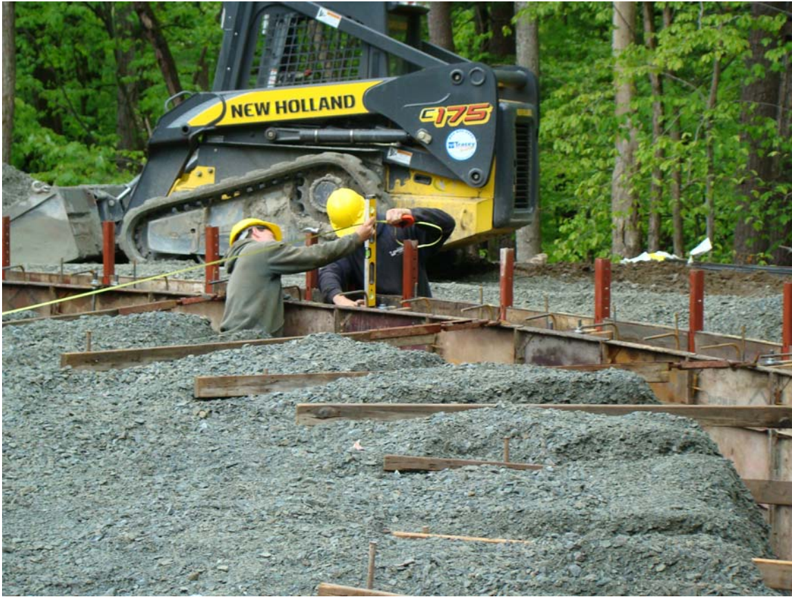
Workers prepare the mold for the circular concrete foundation of the water storage tank in Poestenkill.
